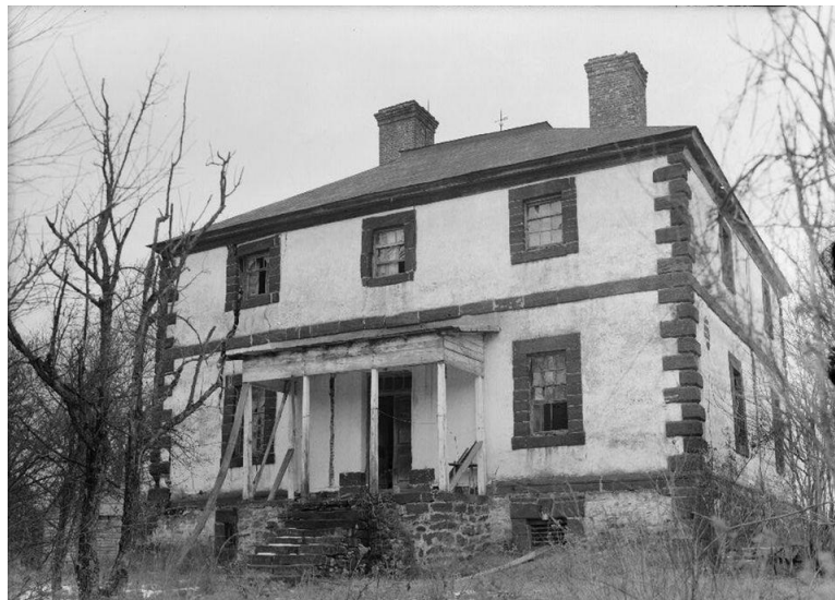
The house at Menokin as it once looked Courtesy of Menokin Foundation
